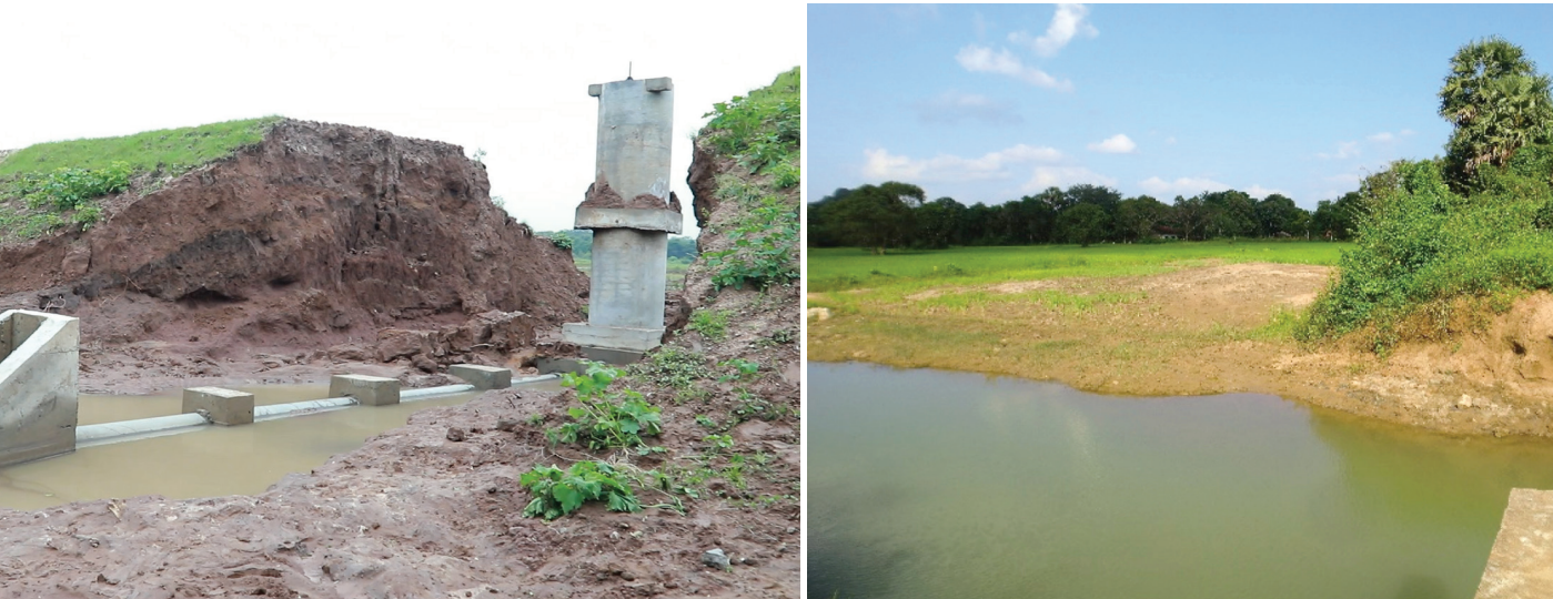
Figure 12: A breached tank due to floods and its effect on agricultural lands
